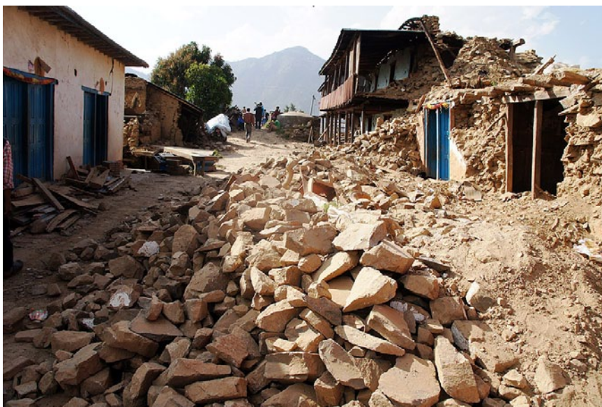
A street in Dhusel village, Lalitpur, which has been entirely destroyed by the April Earthquake. Most people had just started to pick up the pieces when the second tremor hit. Photo: LWF/ C. Kästner
