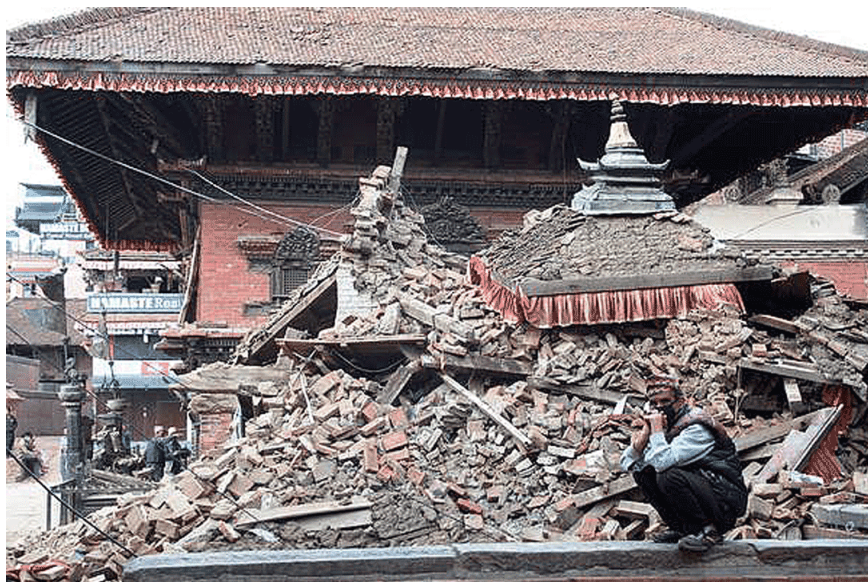
Earthquake destruction in Durbar Square in Bhaktapur, Nepal. Photo: LWF/ C. Kästner
