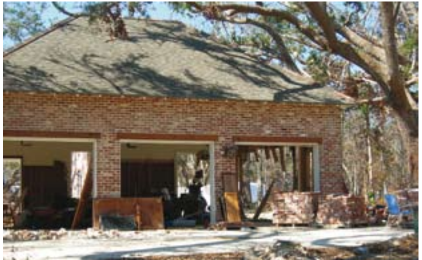
In Ocean Springs, Mississippi, the storm surge carried enough force to smash through the reinforced concrete cement of this garage. © ELCA/M. Nevergall
