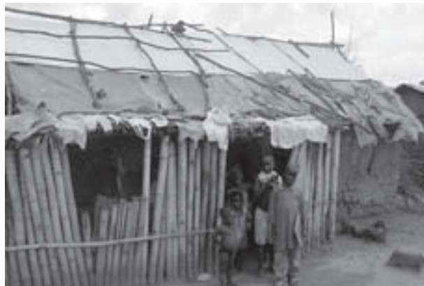
A typical family house at the LWF-run Tobanda refugee camp, in Kenema, Sierra Leone, where thousands of Liberians are residing. The rundown shelters expose families to severe weather conditions. © LWF/DWS Sierra Leone
