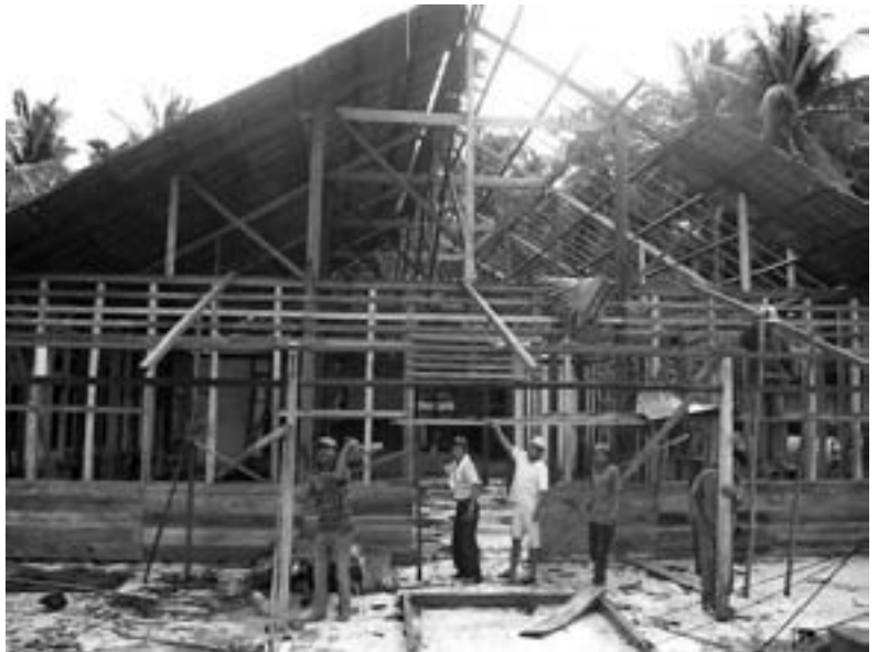
Indonesia, Nias Island: In Sirombu district, community members participate in the construction of the Vabaliwa congregation church, Nias Protestant Christian Church. © Petteri Kokkonen, ACT International/FinnChurchAid
